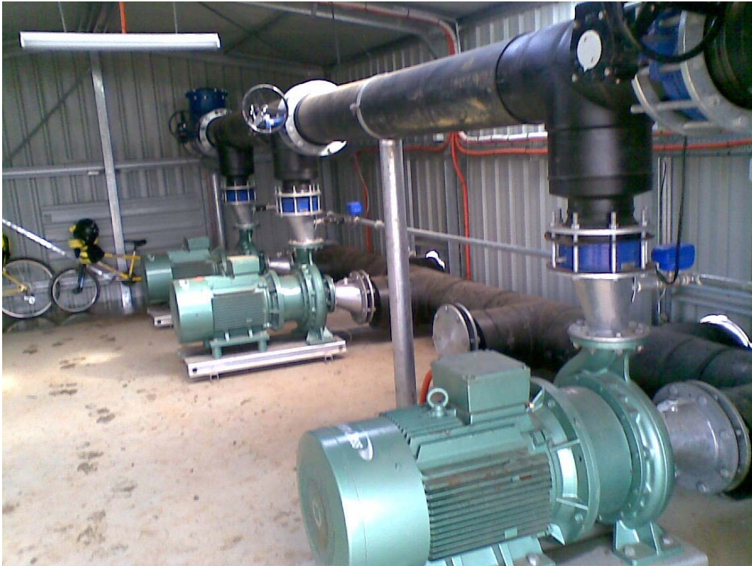
Photo: Three Centrifugal pumps in parallel driven by electric induction motors
